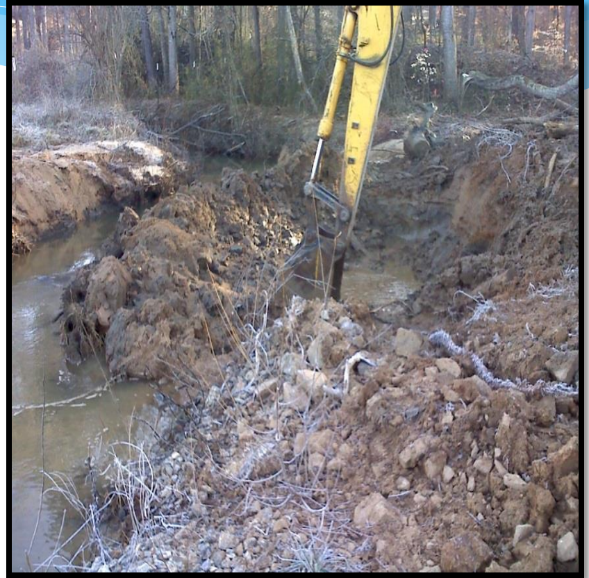
Under-cut creek bed 3 to 4 feet
