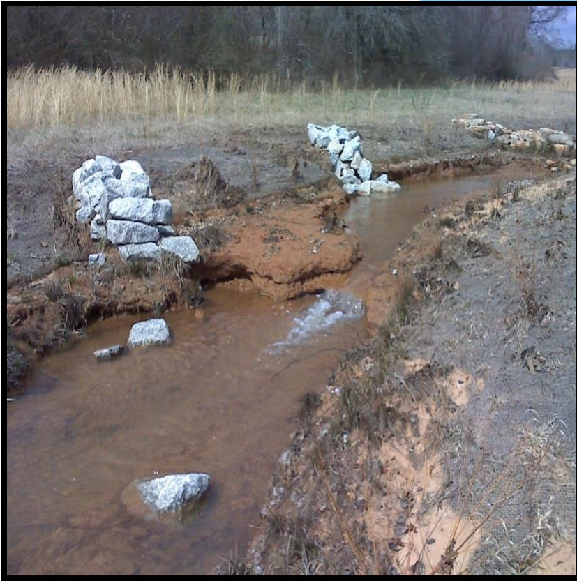
Head Cut Works on Poor Design
