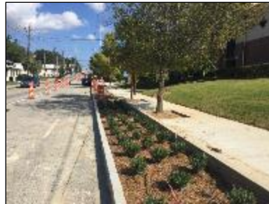
Stormwater Planters Boone Blvd Green Street
